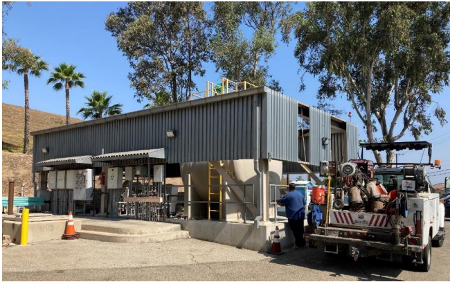
Photograph 7. Sodium Hypochlorite Tank Farm
