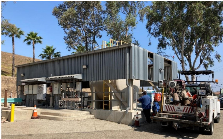
Photograph 3. Sodium Hypochlorite Tank Farm
