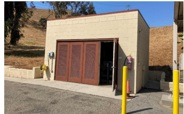
Photograph 6. Backup Generator Enclosure
